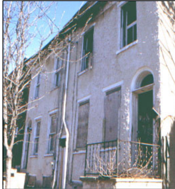
Figure 3.12-3.13: Residential buildings on the east side. The top photo shows 22nd street between Market and Lamotte, where there are many very small buildings in poor repair and problems with crime. The bottom photo show two abandoned buildings on Buena Vista.
